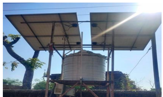
Solar-powered overhead water tank, Bokaro
